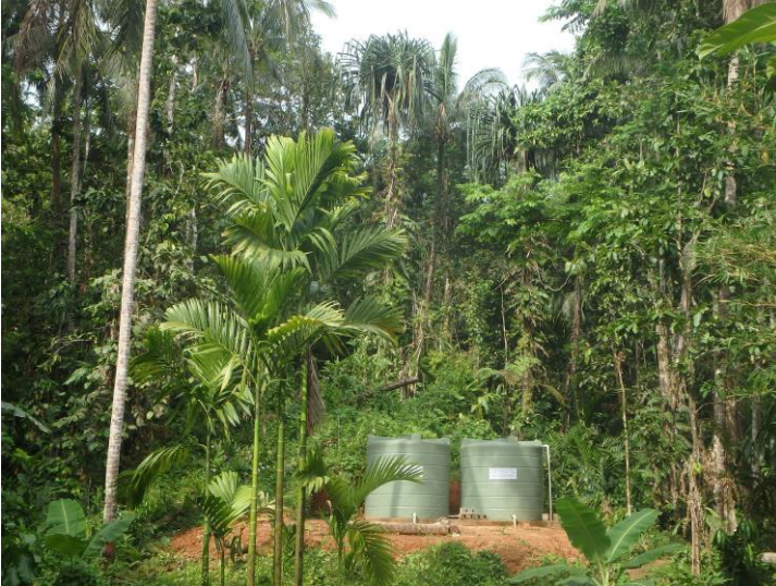
Fig11.Photo: New USAID/SPREP water tanks in Sasamuga, Choiseul
