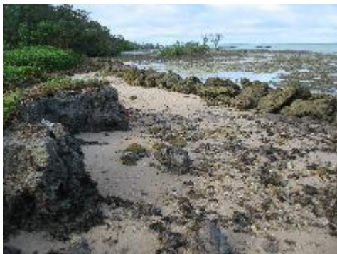
Erosion occurring behind installed rock wall at northern end of Taro airstrip.
