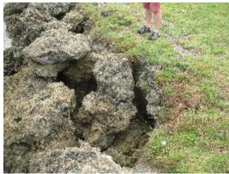
Undercutting adjacent to spaces in the rock wall at northern end of airstrip.
